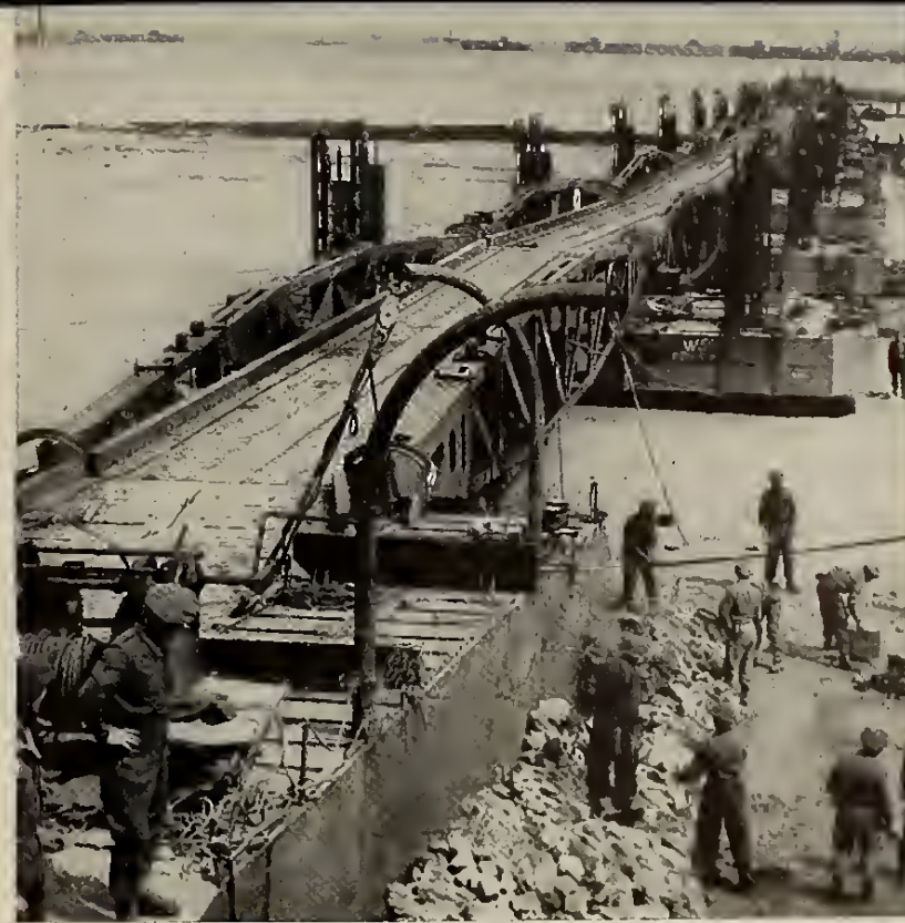
10. Here are seen men of the Royal Engineers putting the finishing touches to the ramp on the Normandy end of the floating roadway. The job of assembling the harbor for U. S. supplies was done by the American Seabees.
